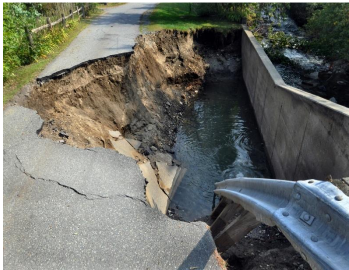
Woodstock, Vt., September 4, 2011 -- Tropical storm Irene caved in many roads after dropping more than 11 inches of rain. This caused floods which destroyed much of Vermont's infrastructure. Photo by Wendell A. Davis Jr.
